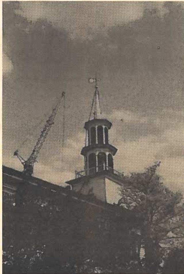
The new steeple and weather vane had just been placed on The Norfield Church before this picture was taken. The old steeple was listing to the rear of the church and there were several decayed timbers which had weakened the whole structure. We have been assured that this steeple will last for at least 100 years.
