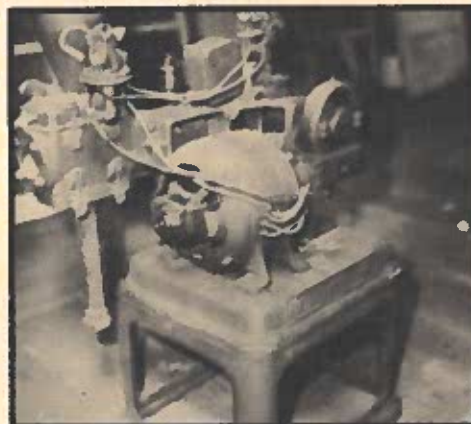
Water pump used on the Fitch property. The pump was made by Kewanee Water Supply Co., Kewanee, Ill. The motor was made by Wagner Electric Manuf. Co. St. Louis, Mo.
