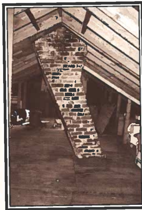
Chimney in attic of house - this was a replacement of a larger central chimney.
