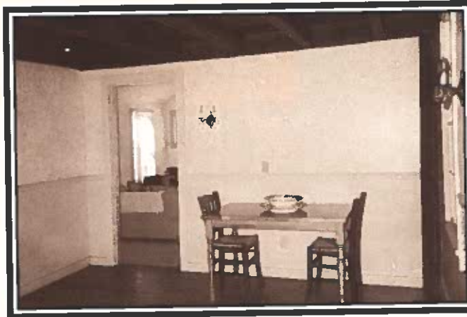
Entry way at 1 Old Mill Road. Ceiling shows original beams with one of 8 support beams showing on right side.
