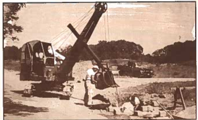
Harold Keene, Herb Gifford and Dave Coley at new drain on River Road
