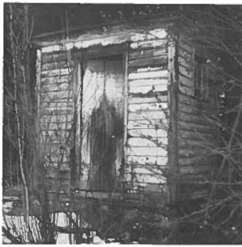
A four-hole outhouse is an original feature of the former Hanford Nichols Estate.
