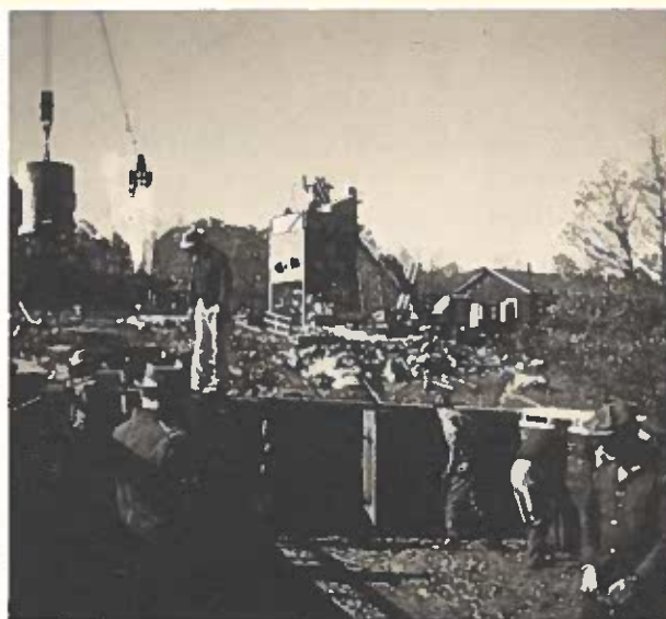
Concrete bucket moving away from dam site after dropping concrete. Saugatuck Dam, Weston.
